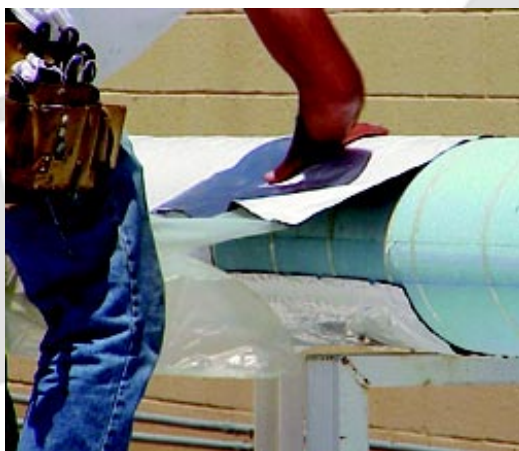
Application of rubberized bitumen vapor retarder/weather barrier membrane on ammonia refrigeration piping system.
