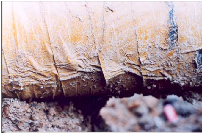
SOIL STRESS FAILURE
