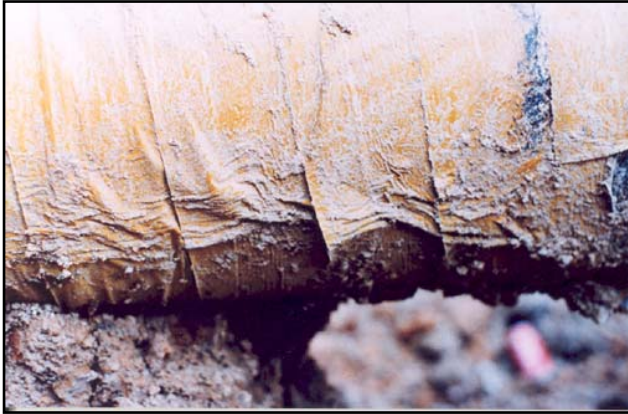
SOIL STRESS FAILURE
