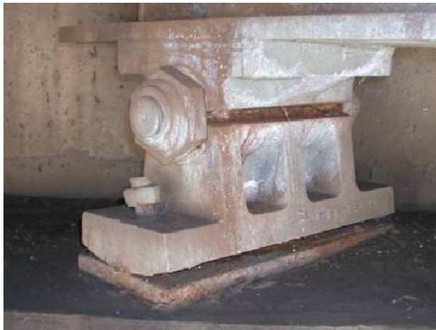
Figure 8 – Uncoated Rocker Assembly Inspection – October 2003
