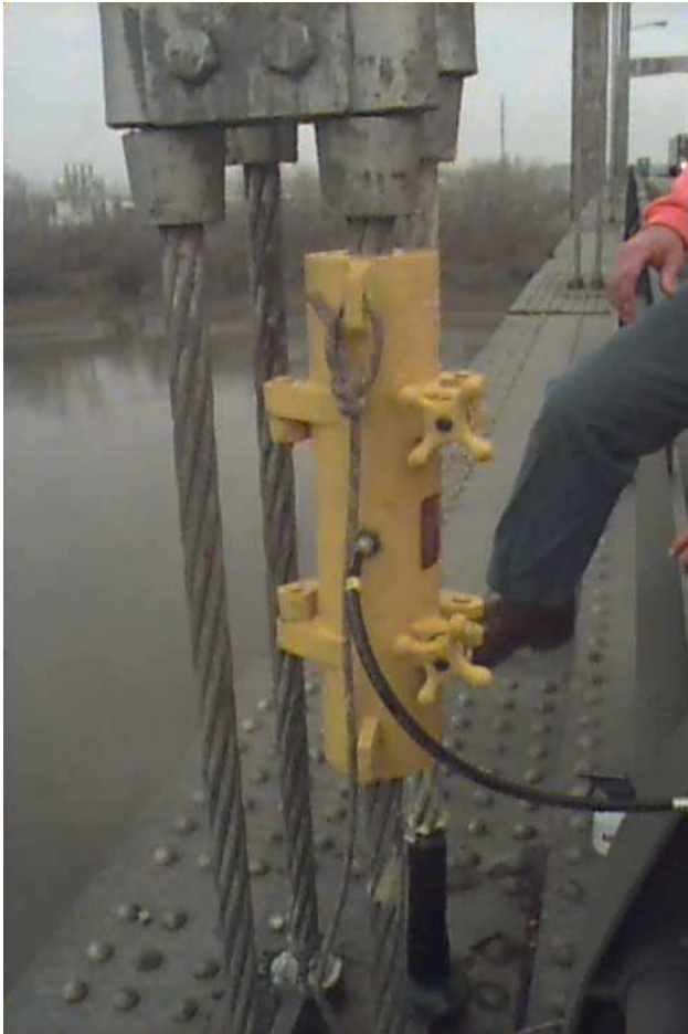
Figure 9 – Bridge Stay Pressure Lubrication – March 2004
